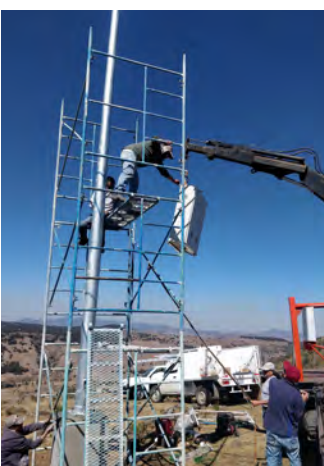
Implementation is carried out by authorized installers and lasts, on average, one day per site.
