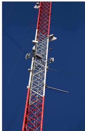
PTP Backhaul Link
