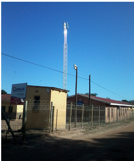
eMMP Access Point tower at school
